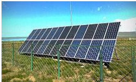
A solar panel with 24 solar modules
